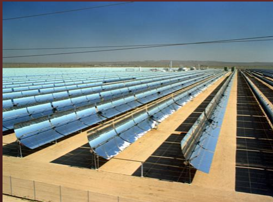
solar electric power plants
